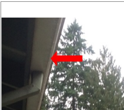
Rain water dripping over gutter edge
