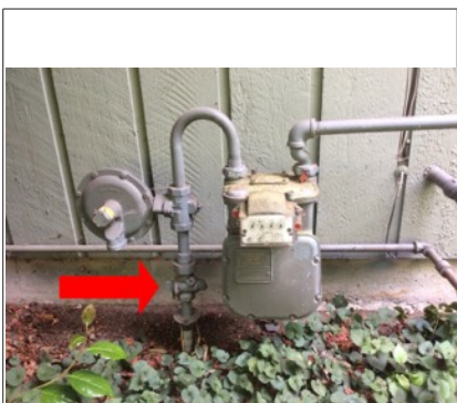
Main fuel shut off located on north side exterior
