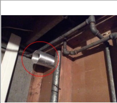
Bathroom vent terminated in adjacent room
