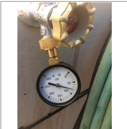
Water pressure measured at 80psi
