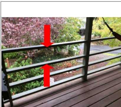
Improper handrail, this is a safety hazard
