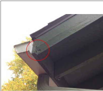
Rotted wood on fascia end at south east corner
