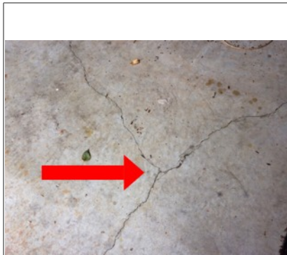
Typical crack at back patio, recommend monitoring.
