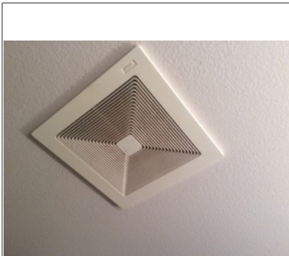
Recommend cleaning vent cover
